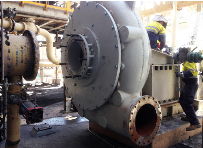
Installation of UMD pump
