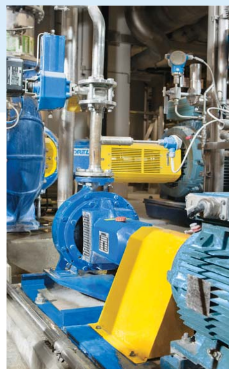
Installed ANDRITZ Pumps ISO Series
